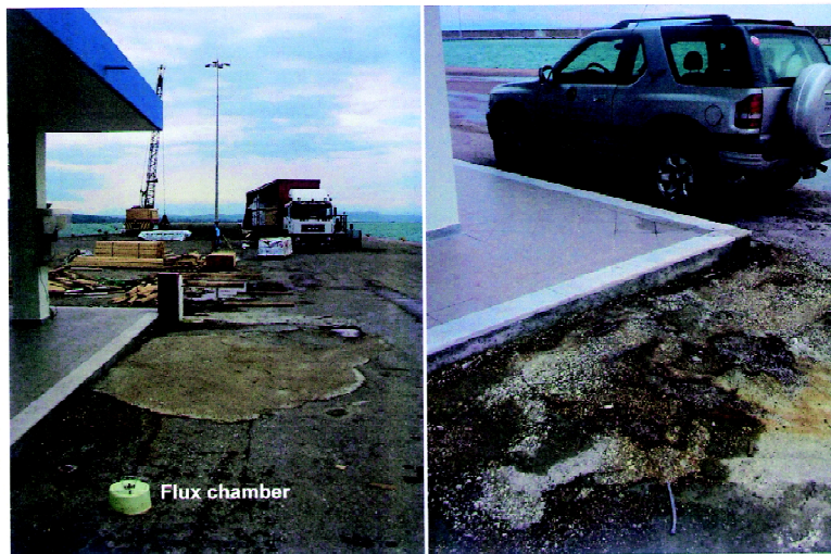
Fig. 5. Seeps in the Katakolo harbour. Left photo: measurement of gas flux (by closed-chamber) from shattered asphalt pavement on the main wharf; a cement plate was spread out to cover the cracks produced by the 1972 explosion. Right photo: H 2 S rich seepage outside of the duty free shop.
